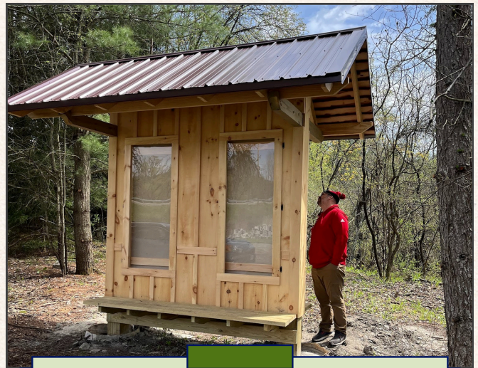
GVSP installed a new kiosk at the Route 305 Trail parking lot in Belfast. Posters/information to come soon.
